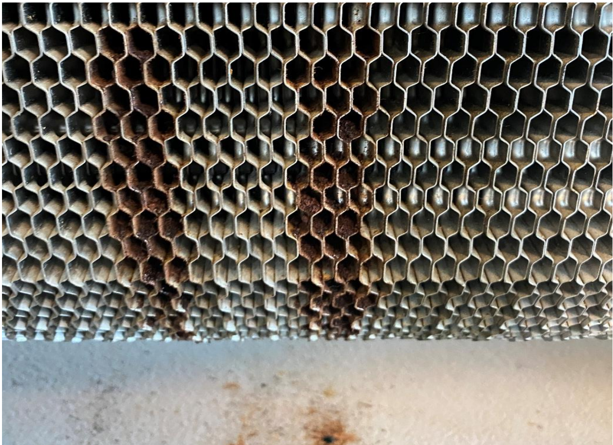
Photo 1 Shows signs of leakage from one of the heat exchangers.
